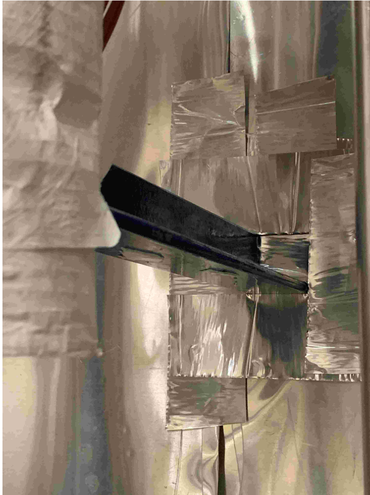
Figure 2.27: Photograph Emphasising L Shape of Support Structure near Value V81 in CIET, Credit Omar Ashraf Alzaabi
