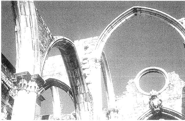
Ruined Gothic vaults of the Cathedral of Carmo, destroyed in the 1755 earthquake and left as a monument.
