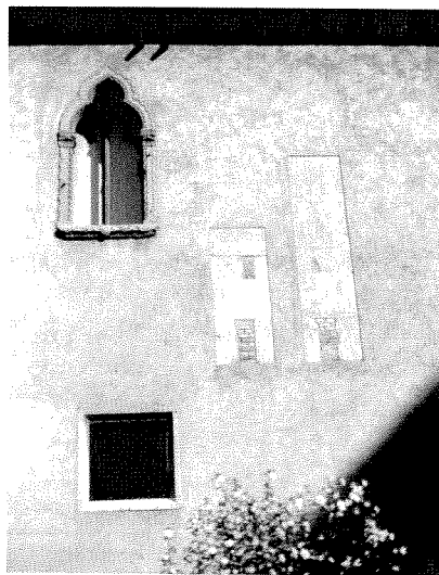
3 Napoleonic and Gothic windows. Also, exterior plaster has been stripped from wall to reveal underlying materials.
