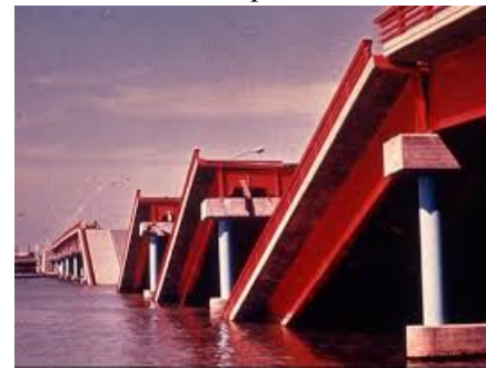
(h) Span collapse and pier failure of the Showa Bridge in the 1964 Niigata earthquake
