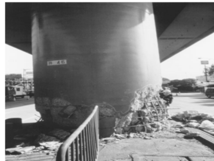
(d) Column shear failure in Hanshin Expressway during the 1995 Kobe earthquake.
