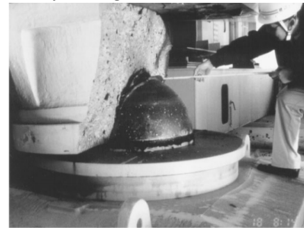
(f) Bearing failure during the 1995 Kobe earthquake.
