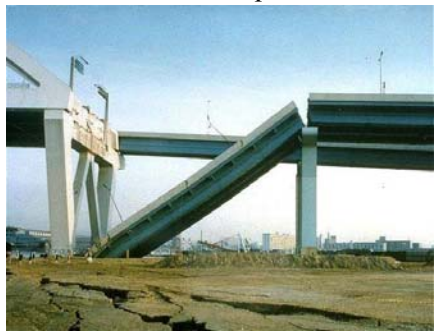
(g) Span collapse of the Nishinomiya Bridge following the 1995 Kobe earthquake
